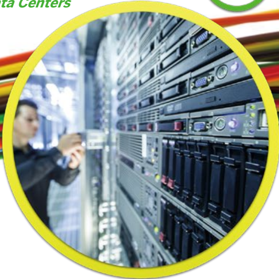
PDU Monitoring for Internet, Financial & Telecom Data Centers
